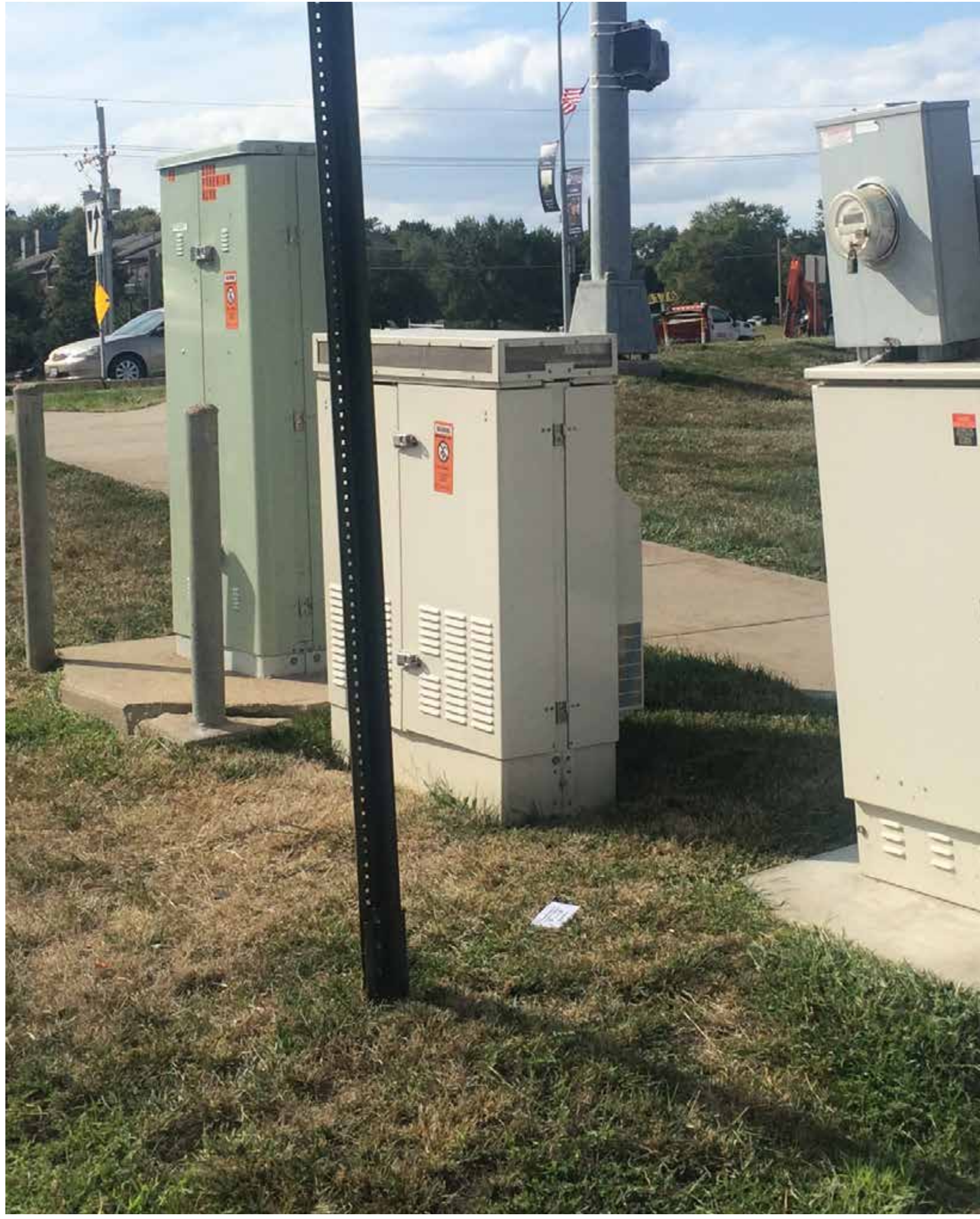
Highly visible utility vaults
